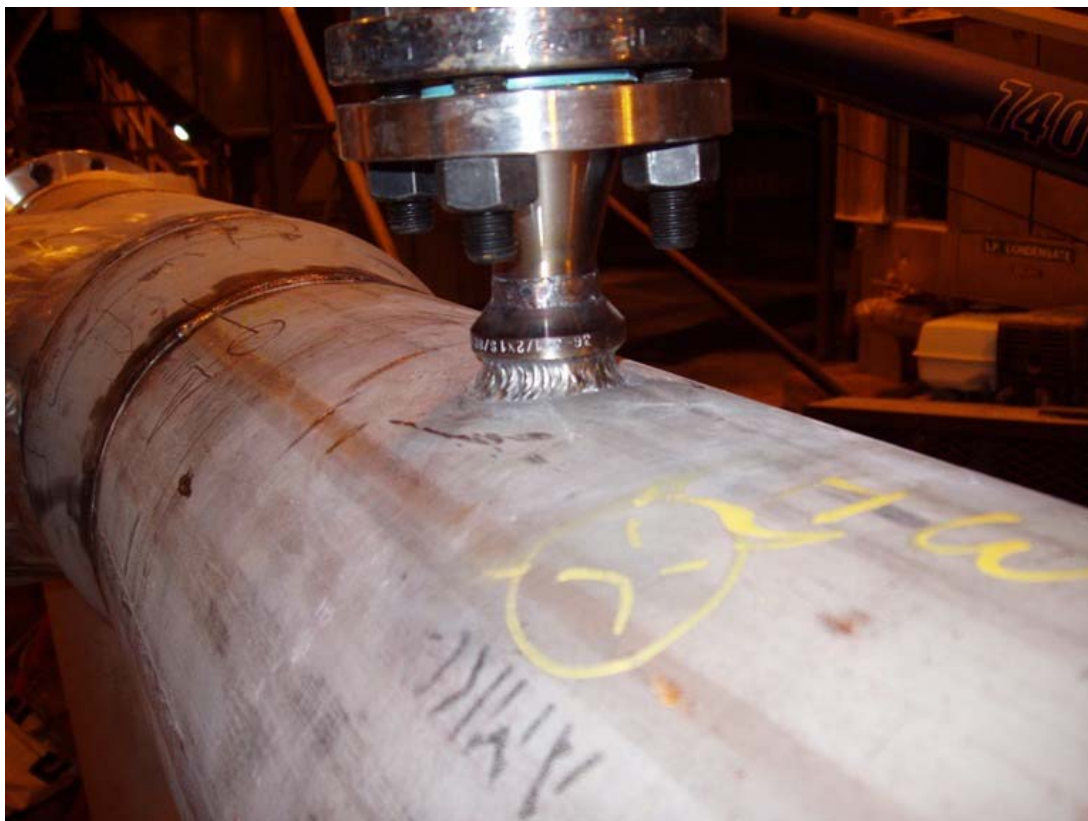
All welds were realized without any defects confirming BHDT's Best Quality and Maximum Reliability. Assuring YARA Canada a Safe and Reliable operation.
