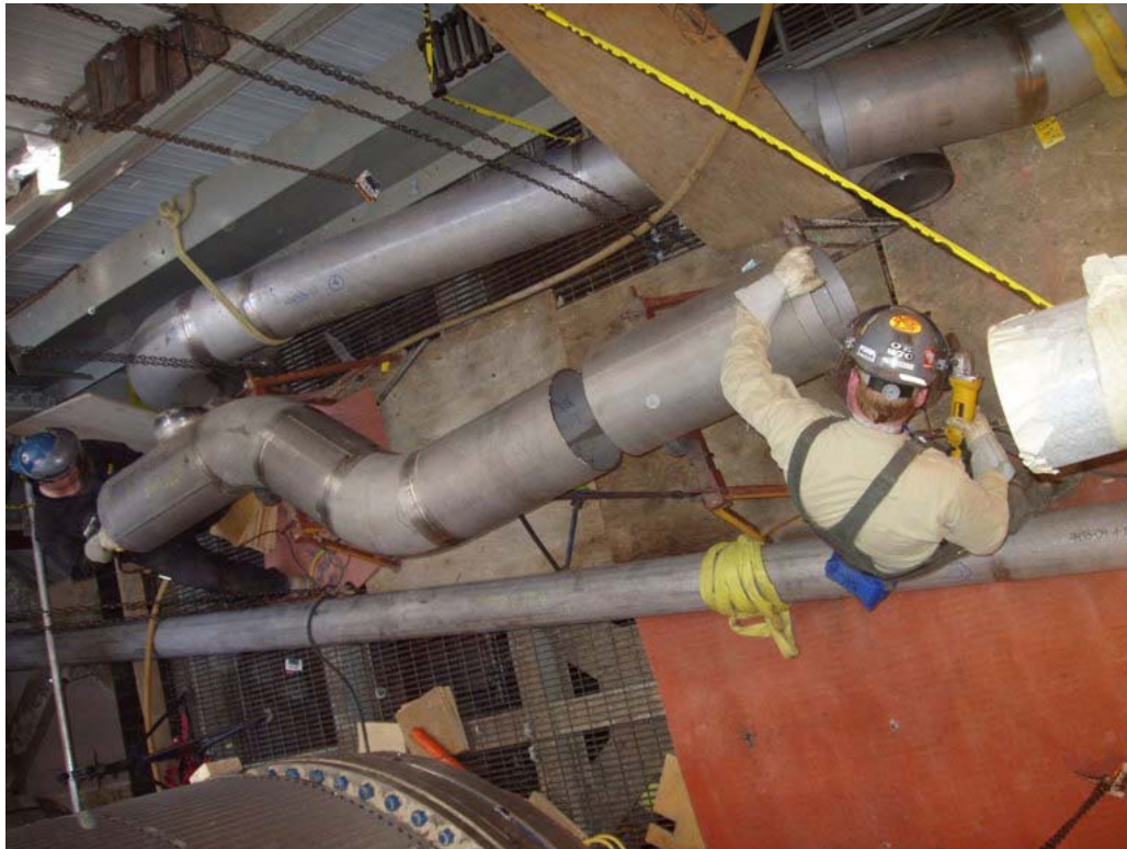
During the turnaround the installation and the remaining welding activities were successfully realized in the limited turnaround period; totally some 150 welds were made and tested.
